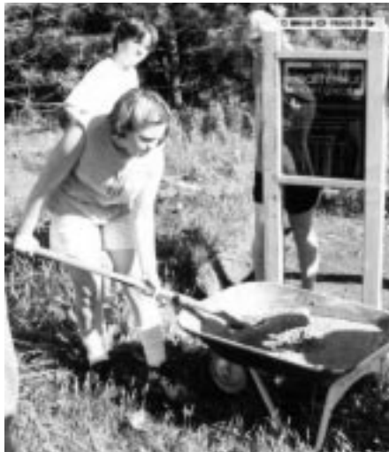
Somerset Students preparing cement to secure a post for a circuit training station.
